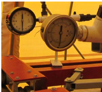
Figure B5. Redundant pressure gauges
