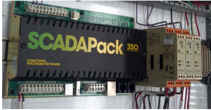
Figure B3. SCADAPack 350 PLC with signal conditioners
