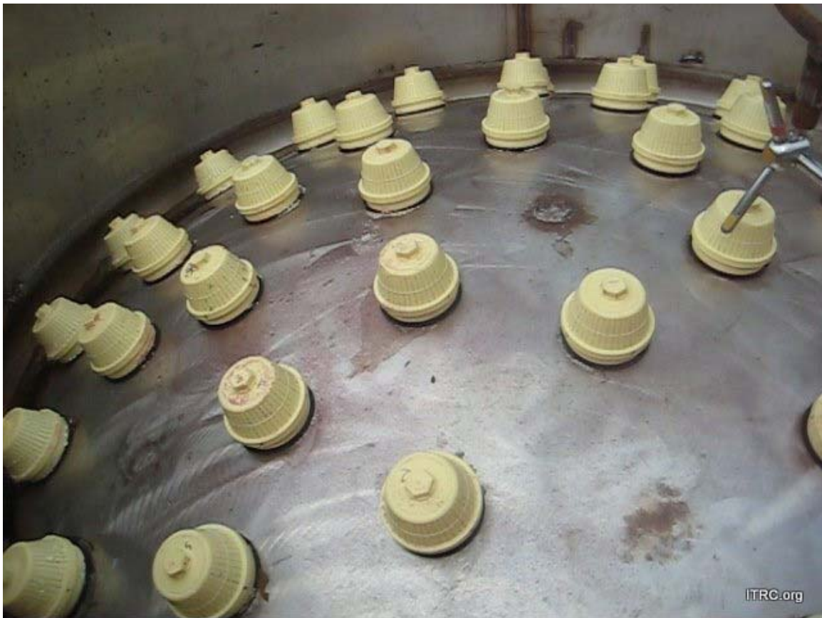
Figure 10. Waterman Dome underdrain. The pods are at different heights, due to the shape of the inverted dome. Photo shows at least 3 locations where pods were expected to be found but were not installed.
